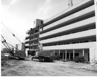
Atlanta Cabana Hotel 1960-2002 Jay Sarno and Jo Harris Demolition Photo: Jon Buono
